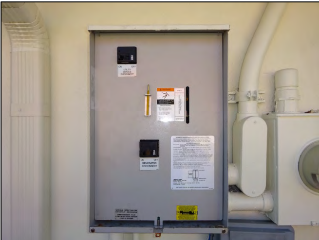
Generac Electrical Panel
