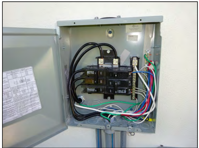
Eaton Electrical Panel
