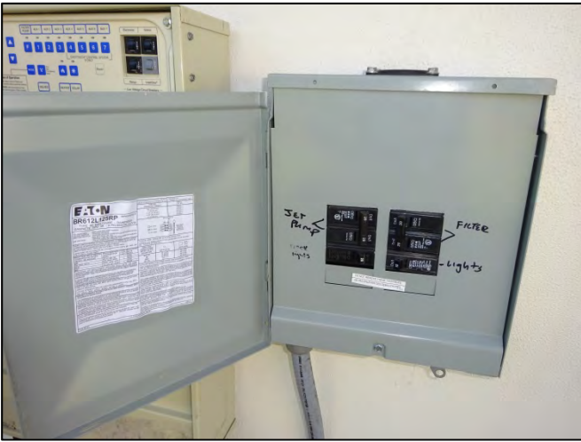
Eaton Electrical Panel
