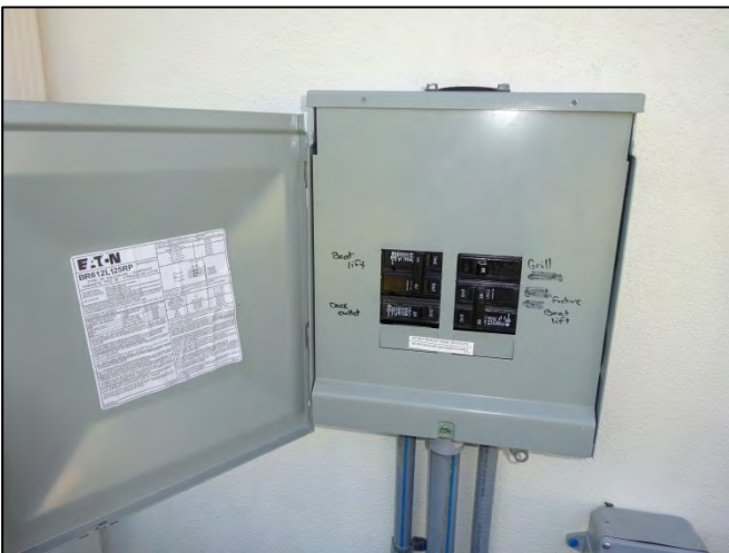
Eaton Electrical Panel
