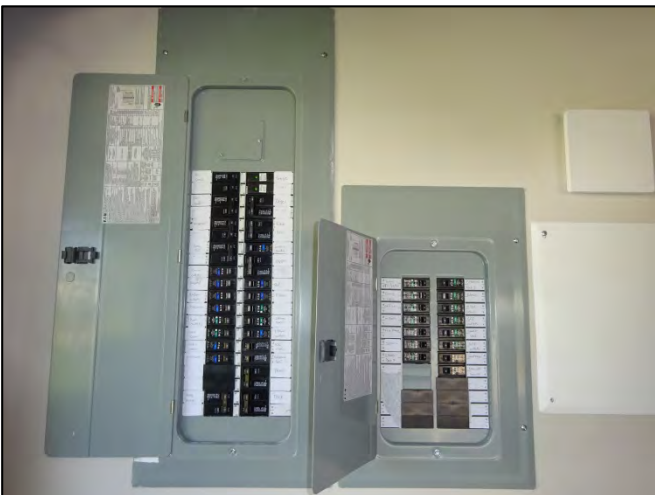
Eaton Electrical Panel
