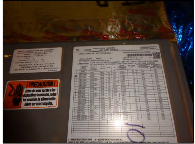
HVAC Label MFD: 08/2018
