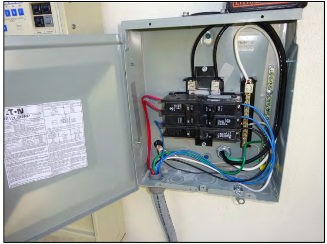
Eaton Electrical Panel
